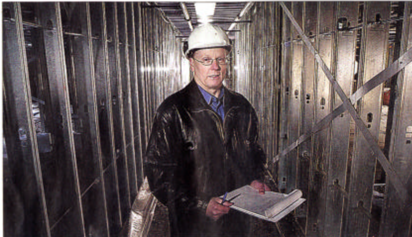
CONDO PROJECT: Martin McLeod, vice-president of business development for Power MBS Structures Ltd., is seen here inside a condominium development under construction in Windsor. The framework of the entire structure is made out of steel.
